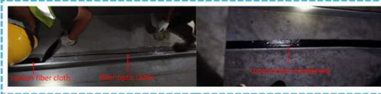
Figure 5. Field installation workflow for the bottom slab sensing cable, including surface preparation, cable pre-laying, material preparation, bonding and protection.
