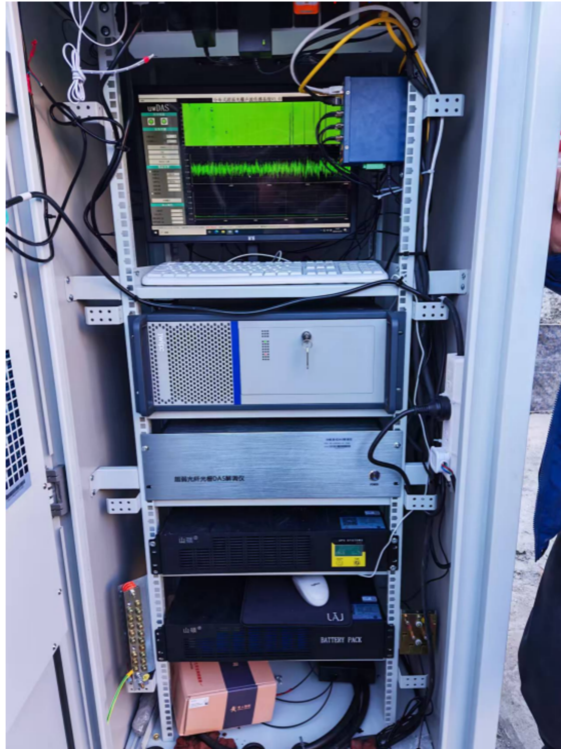
Figure 8. Field cabinet and equipment integration, including DAS acquisition, power, network and supporting devices.
