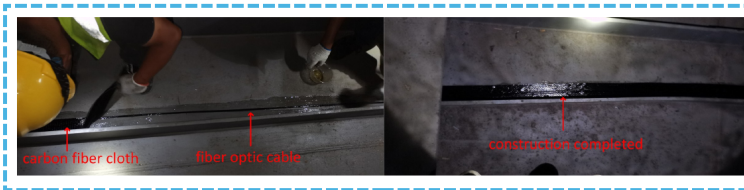
Figure 5. Field installation workflow for the bottom slab sensing cable, including surface preparation, cable pre-laying, material preparation, bonding and protection.
